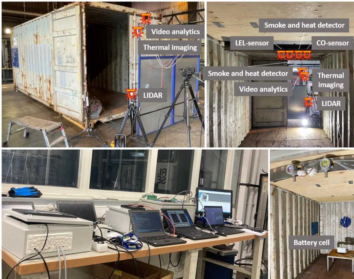
Figure 5. Top left: The container and some of the detectors (outside of the container). Top right: The inside of the container and the location of the detectors. Bottom left: A photo of some of the data acquisition systems. Bottom right: A free-standing battery cell and detectors on the ceiling inside the container.
