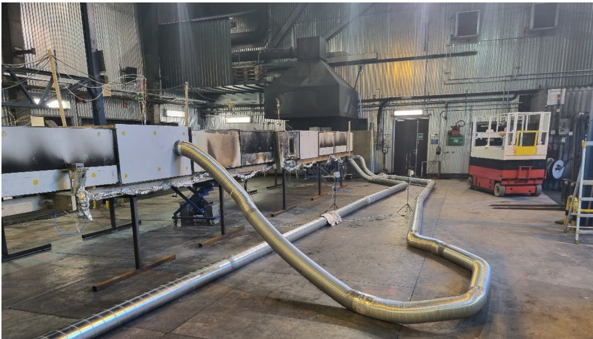
Figure 30: Duct from the model to the hood for measurement of HRR. Exhaust fan in section 8 (closest).
