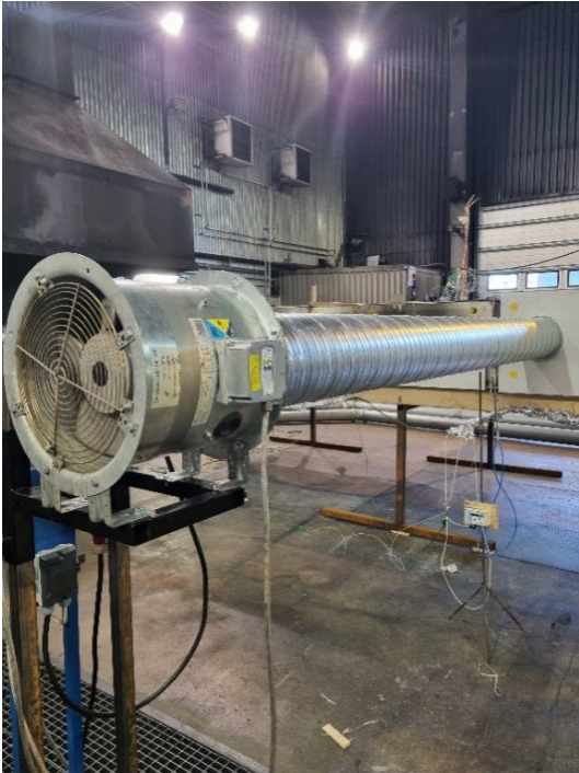
Figure 29: Supply fan in section 4.
