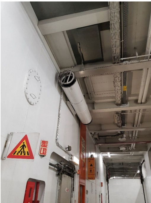
Figure 3: Jet fan on deck 3
