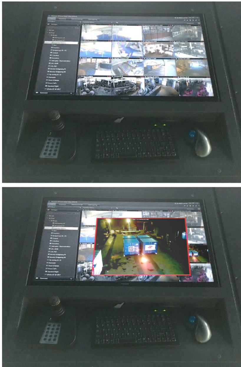
Figure 4: CCTV panel from Pearl Seaways (left) and imagined presentation of the alarm information via highlighting the CCTV from fire area. The flame and smoke boundaries may also be highlighted by the detection system as shown in Figure 31.
