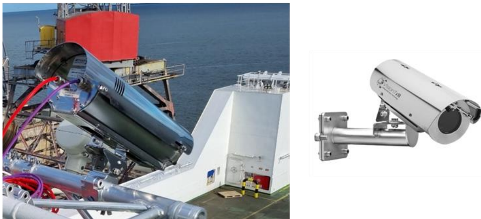
Figure 7: Example thermal imaging (infrared) camera installed on board Hollandia Seaways for LASH FIRE evaluations.
