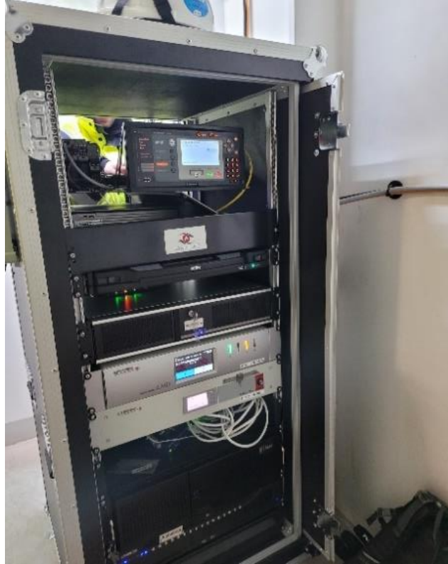
Figure 58: LASH FIRE box on board Hollandia Seaways containing a fire alarm panel, draw-out monitor and keyboard, several computer cases, some data acquisition systems, and associated accessories.
