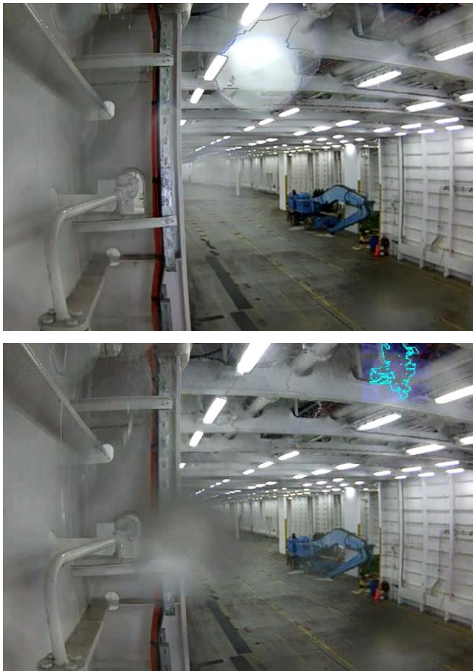
Figure 56: Nuisance alarm example from the video fire detection system in the closed deck during washdowns: the droplets landing and moving on the lens of the camera are misinterpreted as smoke (boundaries highlighted using grey and blue contours in mid-top and top right of the two pictures, respectively).
