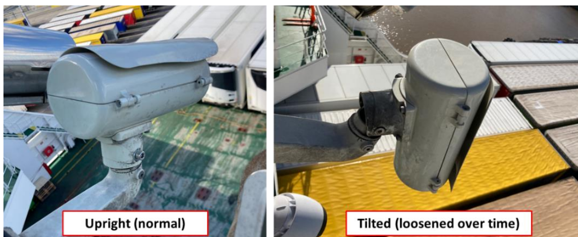
Figure 57: Camera tilting observed due to the connections getting loose over time.
