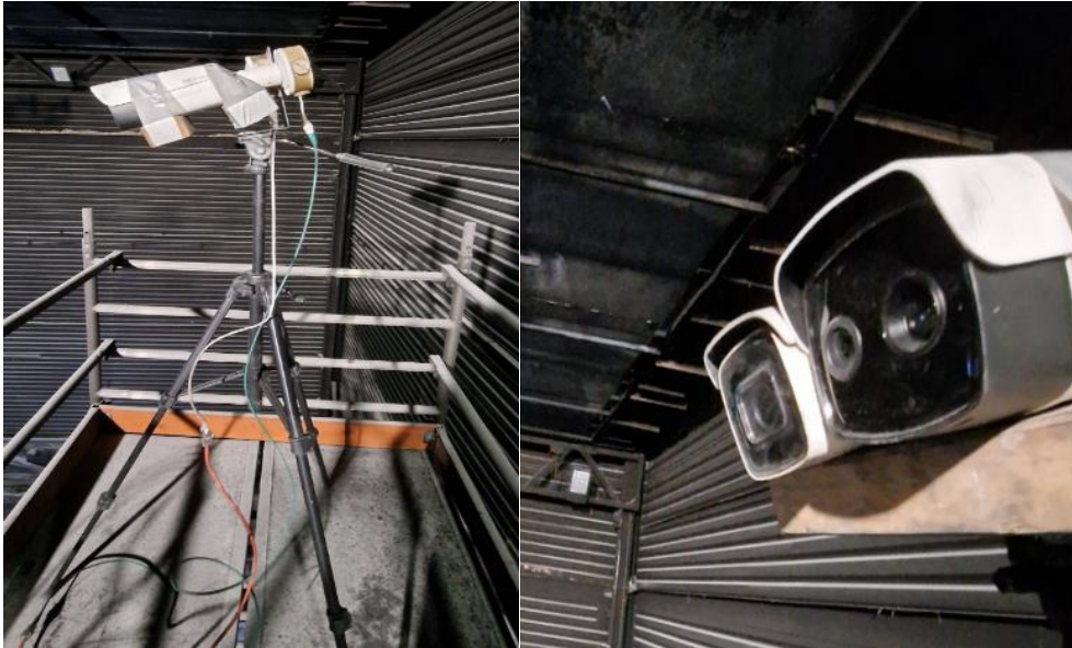
Figure 40: Thermal imaging (IR) camera and regular CCTV camera installed at 10 m height and 27.1 m horizontal distance from the burner shown in Figure 39.
