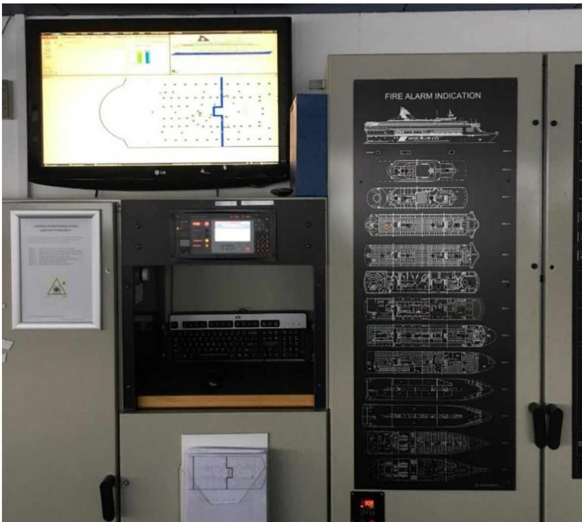
Figure 3: Fire detection panel on Pearl Seaways.
