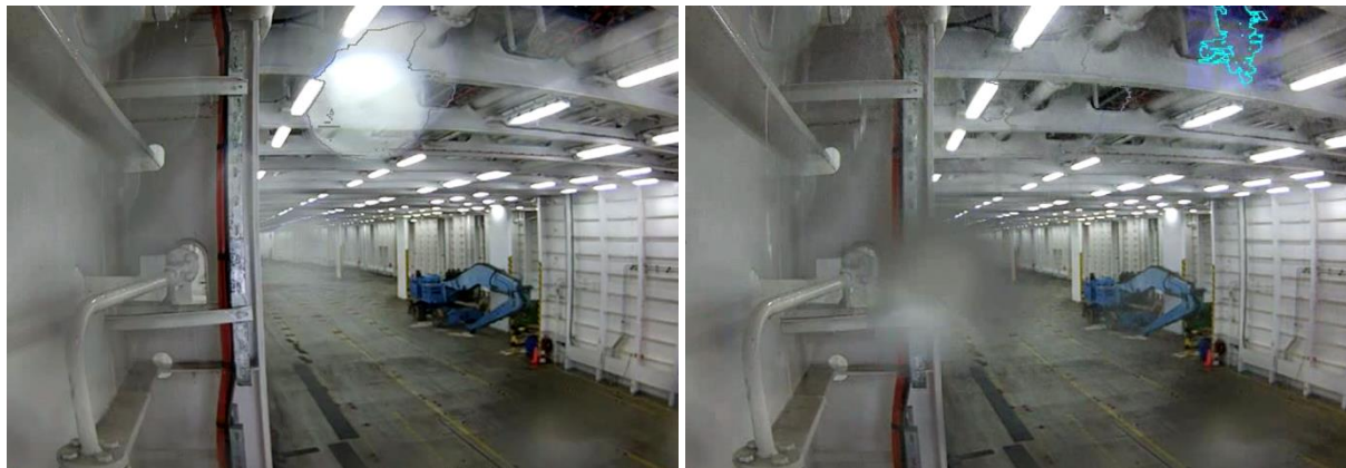
Figure 45: Nuisance alarm example from the video fire detection system during washdowns: the droplets landing and moving on the lens of the camera are misinterpreted as smoke (boundaries highlighted using grey and blue contours in mid-top and top right respectively).
