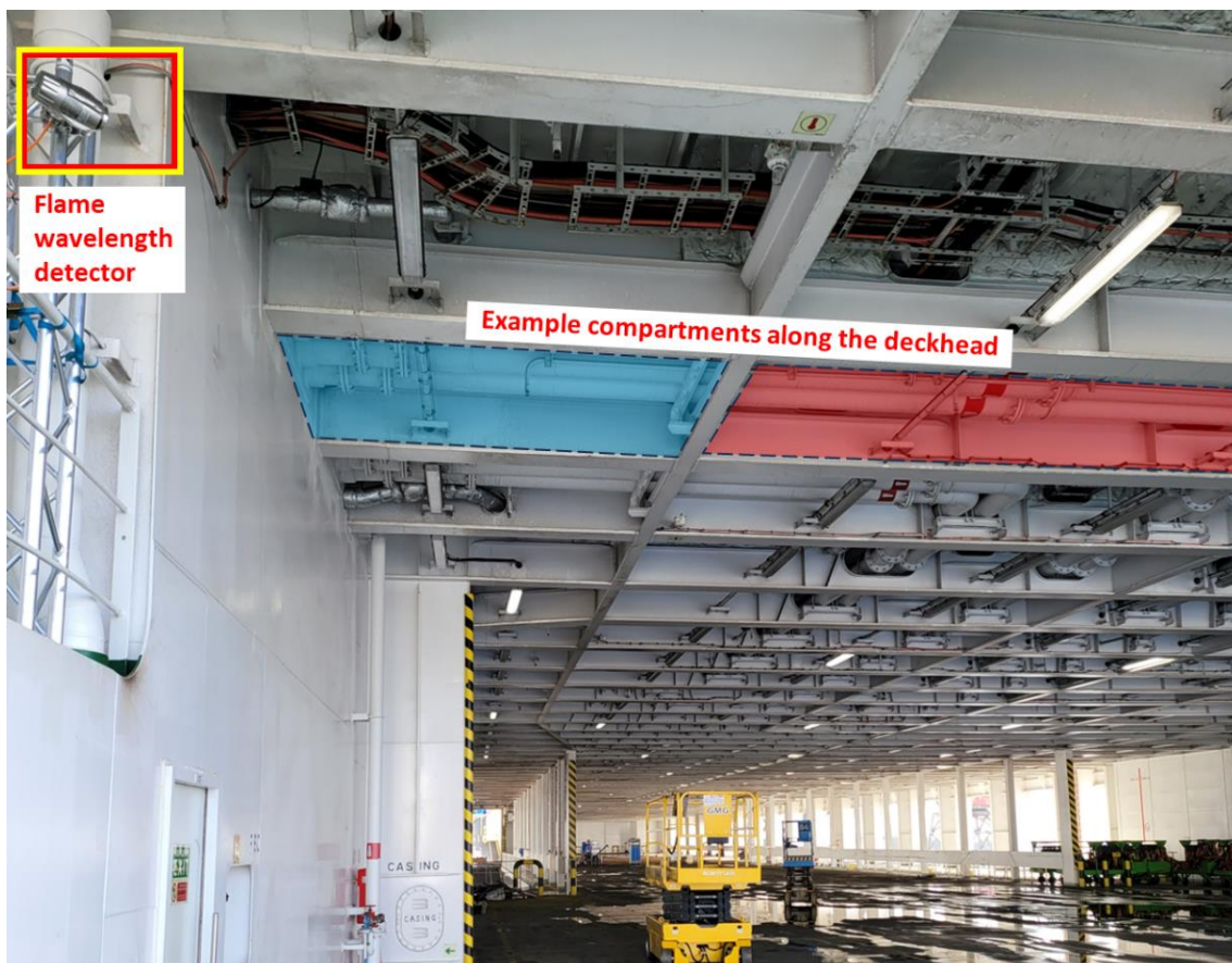
Figure 41: Triple-IR flame wavelength detector installed on Hollandia Seaways for the LASH FIRE trials. The photo also shows examples of compartments along the deckhead which are arranged as shown in Figure 37.
