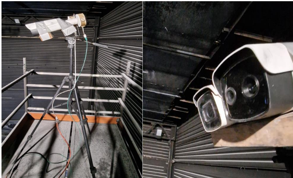
Figure 32: Thermal imaging (IR) camera and regular CCTV camera installed at 10 m height and 27.1 m horizontal distance from the burner shown in Figure 31.
