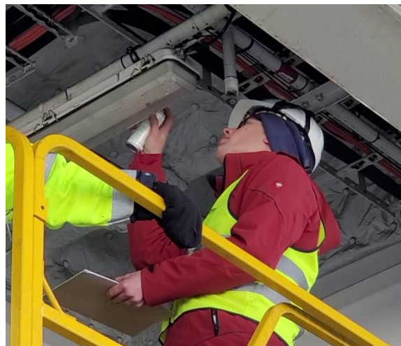
Figure 38: System expert using a frost spray to pinpoint the locations of the different rows of fibre-optic cables installed along the deckhead.
