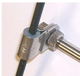
Figure 55: Example sensor cable installation with a steel clamp (DIN 3016) with a reduction sleeve for thermal insulation.
