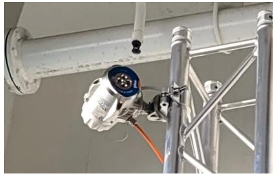
Figure 2: Example flame wavelength detector unit installed on board Hollandia Seaways for testing. The orange cable connects the detector to the fire control panel where the alarm signal is received and processed.
