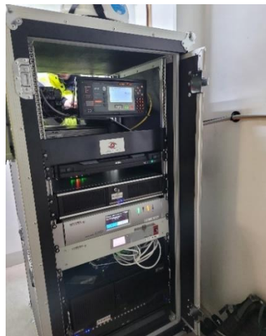
Figure 39: LASH FIRE box on board Hollandia Seaways containing a standalone fire alarm panel, draw-out monitor and keyboard, several computer cases, some data acquisition systems, and associated accessories.
