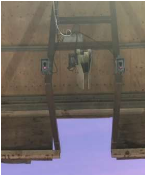
Figure 6 Front ANPR cameras, facing south in the gate house. (STL)
