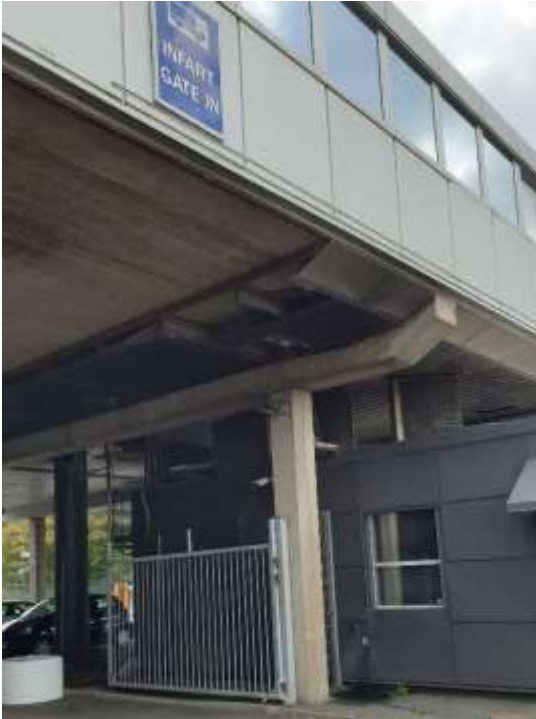
Figure 7 Front edge of office building in front of the gate to the south.
