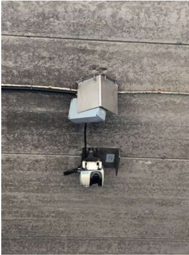
Figure 21 Damage to junction box at Majnabbe. (STL)
