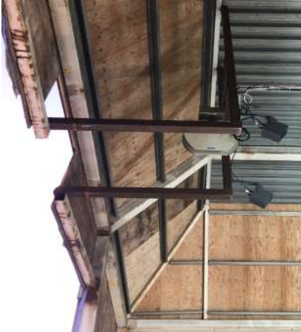
Figure 12 Second LiDAR plus forward license plate readers at the exit of the gate house.
