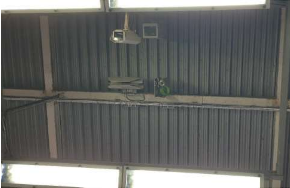
Figure 14 Vertical installed LWIR and LiDAR (RISE)
