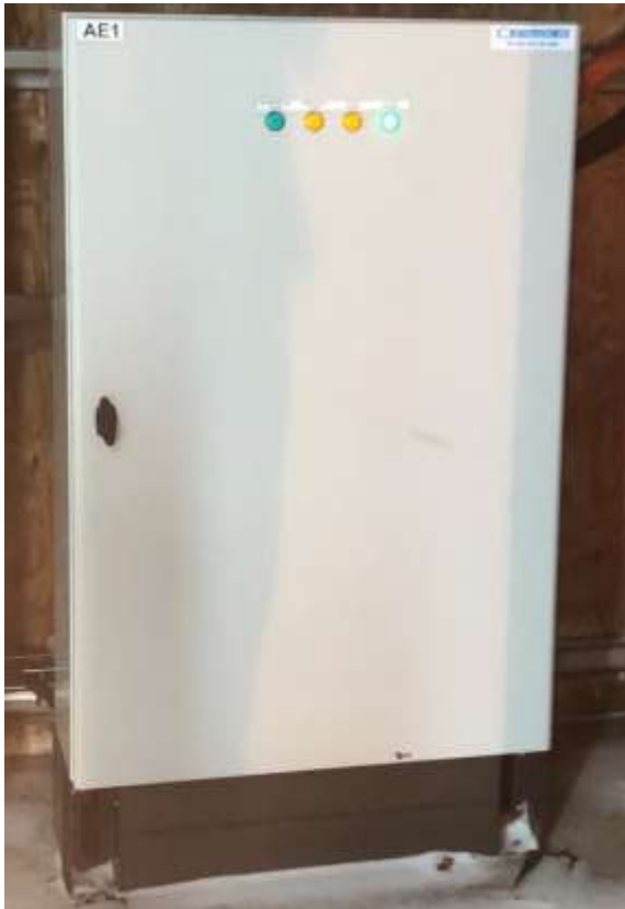
Figure 18 VHD system cabinet. (STL)
