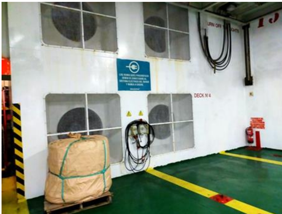
Figure 2 - Picture from ship BAHAMA MAMA-BALEARIA of mechanical ventilators
