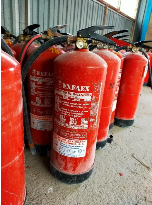
Figure 10. Dry Chemical powder extinguisher.
