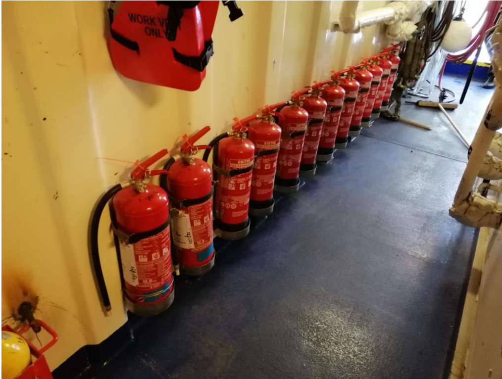
Figure 10. On-board disposal of hand-held (lighter than 20kg) portable fire extinguishers
