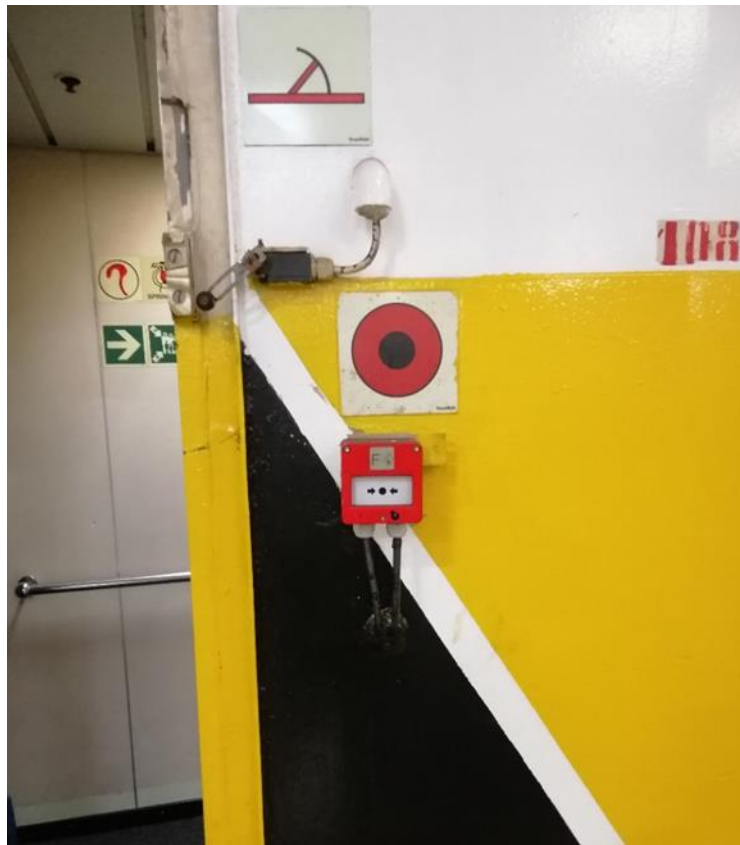
Figure 9. Manually Operated Call Point for raising the fire alarm. Ro-pax NAPOLIS January 2020
