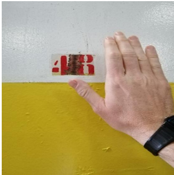
Figure 4. Framing marks on bulkhead. Difficult to read.
