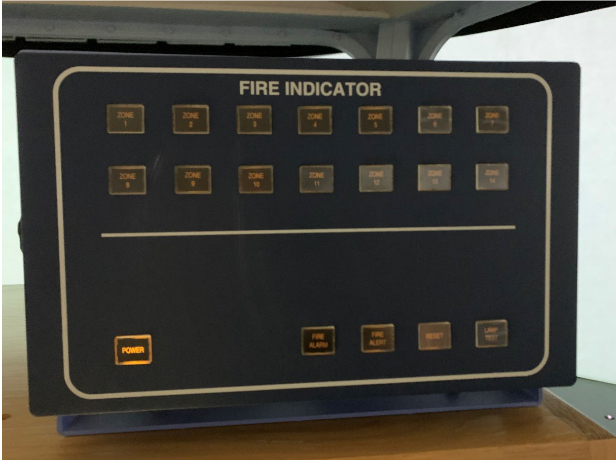
Figure 10 Fire alarm panel on the simulated bridge
