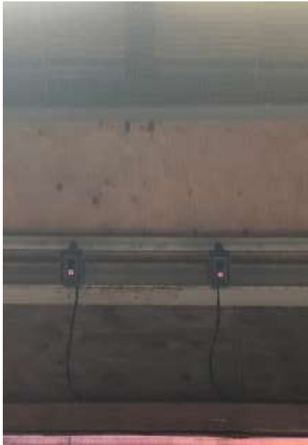
Figure 7 Two rear license plate cameras mounted in the south side ceiling. (STL)
