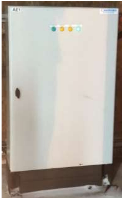
Figure 10 Exterior of TEMS cabinet. (STL)
