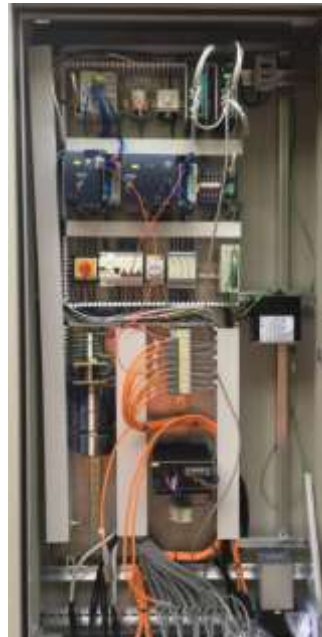
Figure 11 Interior of a TEMS cabinet. (SICK)
