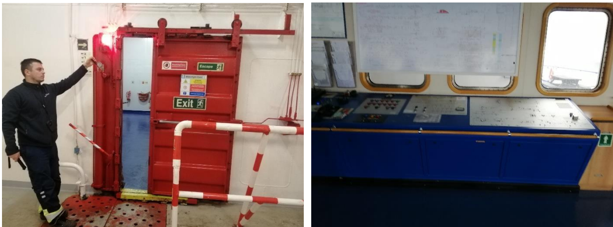
Figure 3 - Pictures from trip onboard Stena-Flavia (water tight door + control room)
