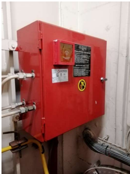
Figure 16. Release box for control of activation of the CO 2 system. BALEARIA ro-pax vessel.
