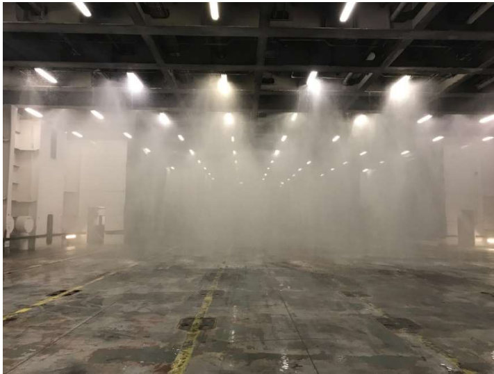
Figure 2. Active drencher system on a car deck.
