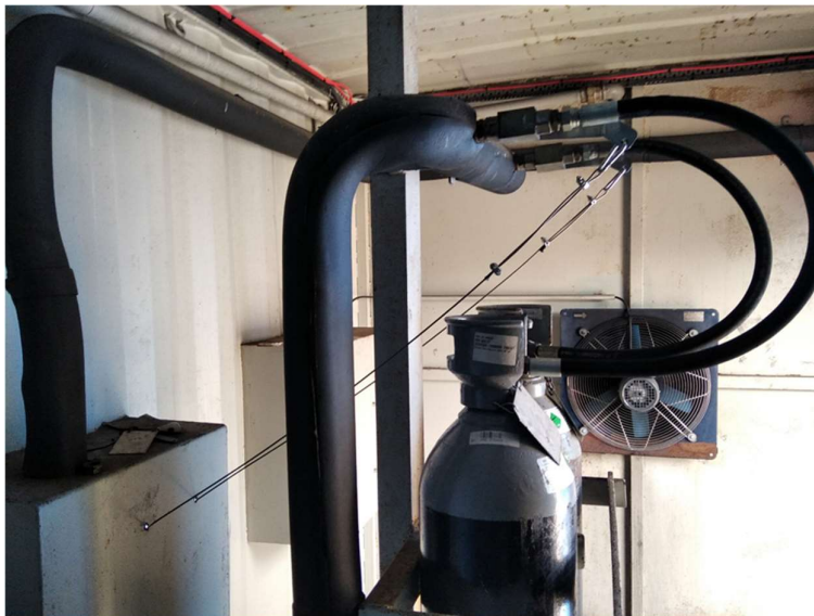
Figure 23. CO 2 cylinders and ventilation
