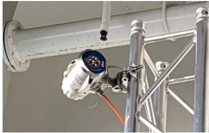
Figure 8: Example flame detector unit installed on board Hollandia Seaways for testing. The orange cable connects the detector to the fire control panel where the alarm signal is received and processed.
